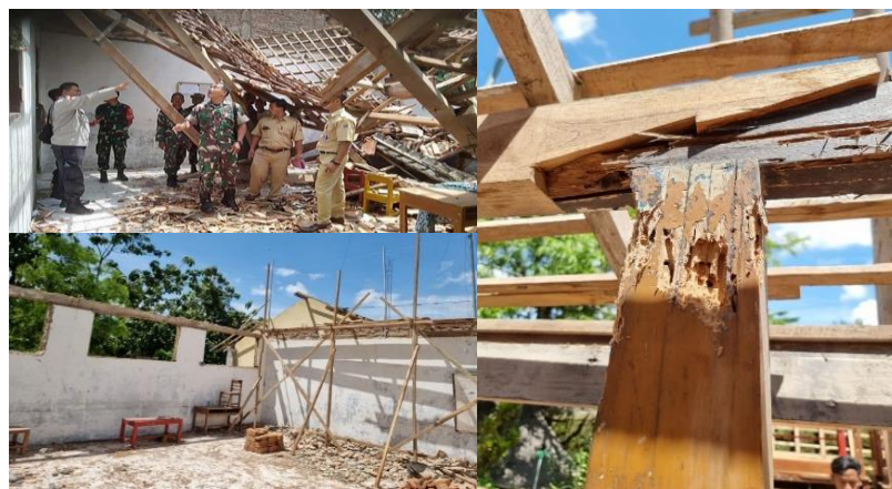
Figure 1. MI Muhammadiyah Gemantar Mondokan Building After the Roof collapsed.
