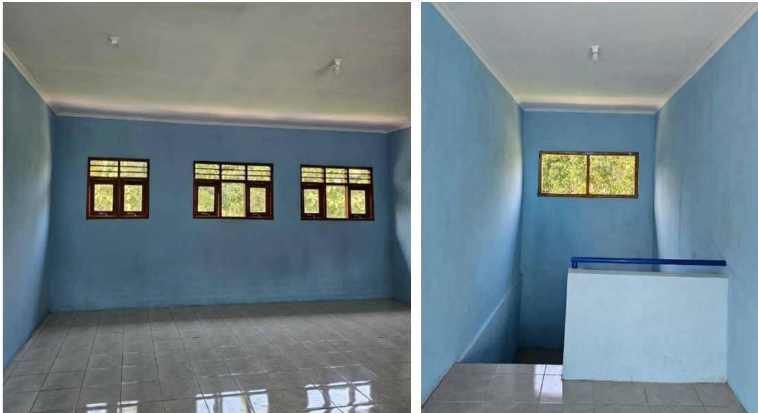
Figure 5. Light Points in the New Classroom and Installation of light points in the stair area to the 2 nd floor
