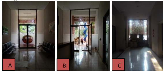
Figure 2a. Some Damp and low light areas in the corridor on the 1 st Floor (A, B,C)
