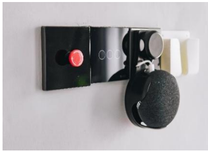
Figure 2. Installation of Google Nest (Source: Author's Document, 2025)
