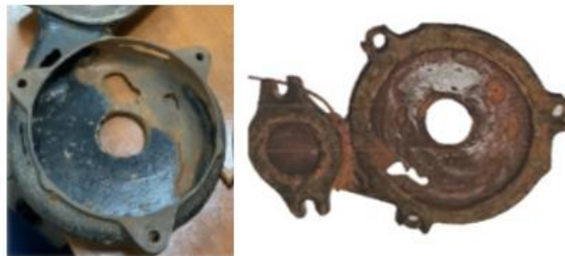
Figure 2. Condition of the pump casing after damage
