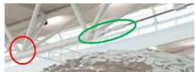
Figure 2. The joint construction of the KJT roof uses a combination of welded and pin.
