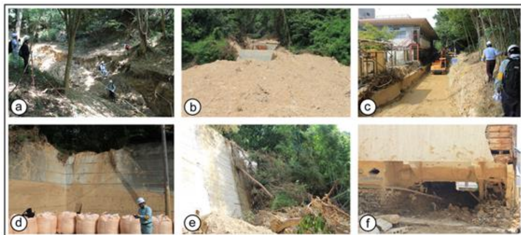
Figure 2. Photographs of the 2018 heavy rainfall event that triggered (a) erosion in the hills, (b) destroyed a check dam in the Sumiyoshigawa River, (c) eventually flowing down to the dwellings of Kobe City by (d) overtopping protection walls and (e) check dams, eventually filling houses with sediments, blocks, and driftwood (f).
