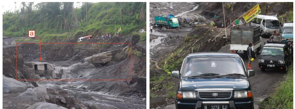
Figure 14. Damage impact on the Sabo DAM (left) and the disruption of road access in Supiturang Village, Pro-nojiwo District, Lumajang Regency (right). Note: (a) Damage to the SABO DAM
