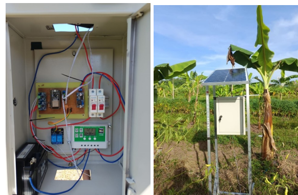
Figure 4: Tool placement: (a) Inside the box panel, (b) In the field
